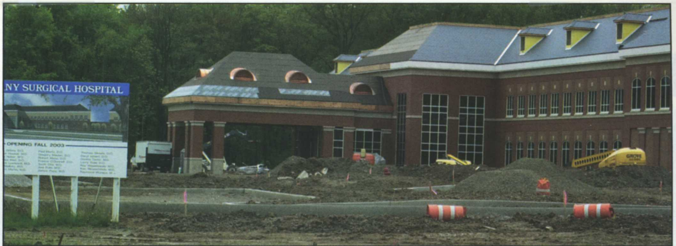
New Albany Village Administrator Joseph Stefanov says he's interested in seeing medically related development around the still-under-construction New Albany Surgical Hospital.
